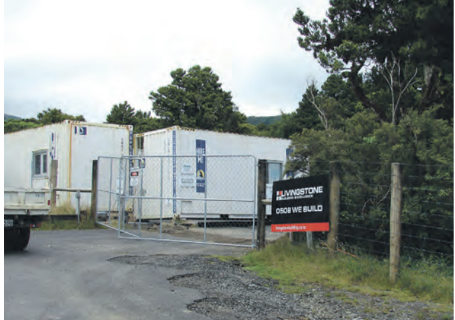
Prefabs are on site in readiness for construction of the new accommodation facility.
